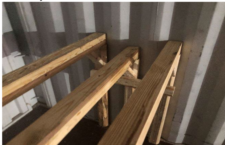
Fig 2. Lumber cradle construction to support the axel of an upper tier vehicle.
