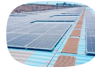
APM Terminals Pipavav, India, 1 MW rooftop solar at the terminal
